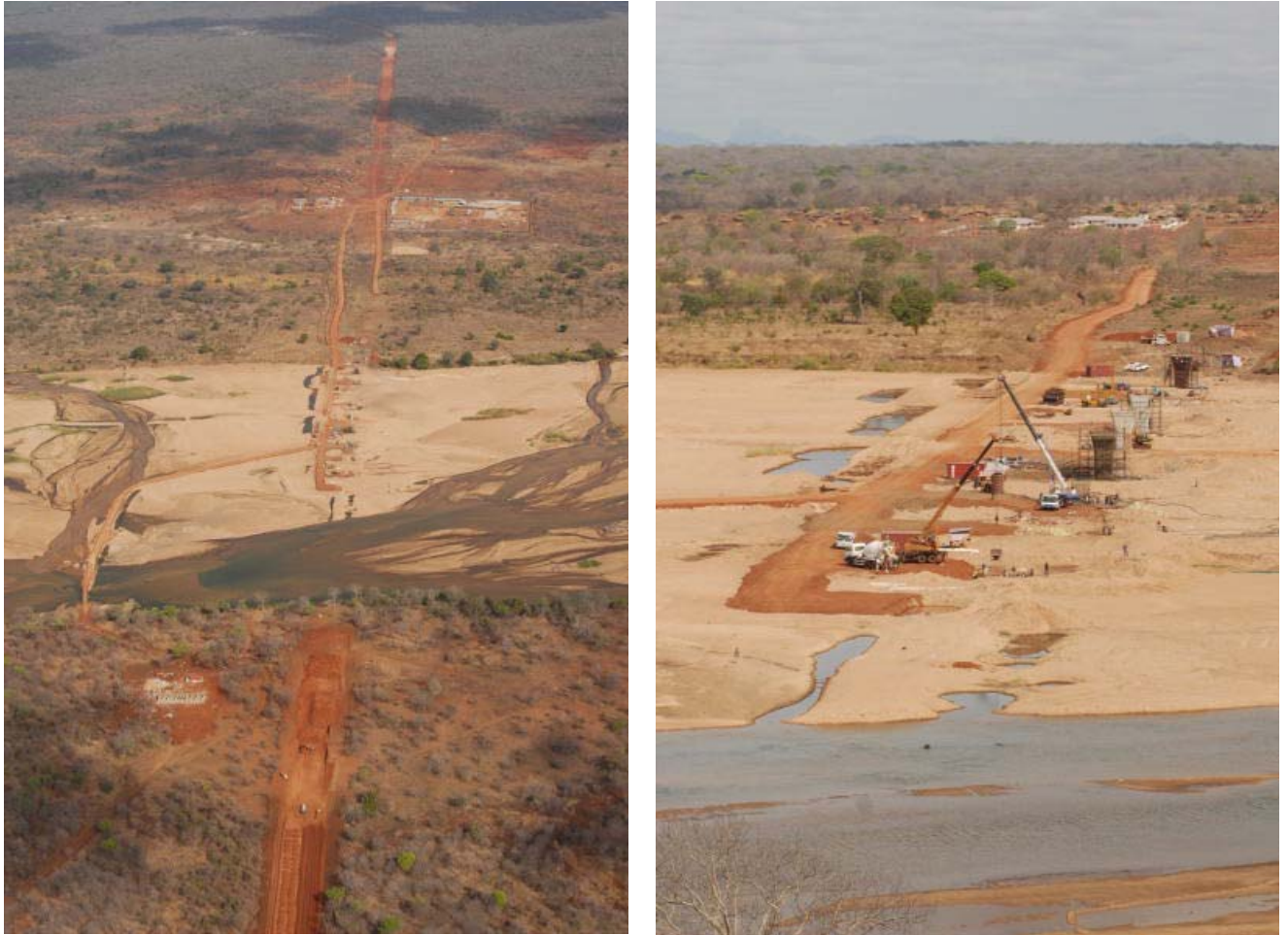
Fig 23: Construction of Freedom bridge over the Rovuma River in north-eastern NNR which will link Tanzania and Mozambique –Nov 2006
